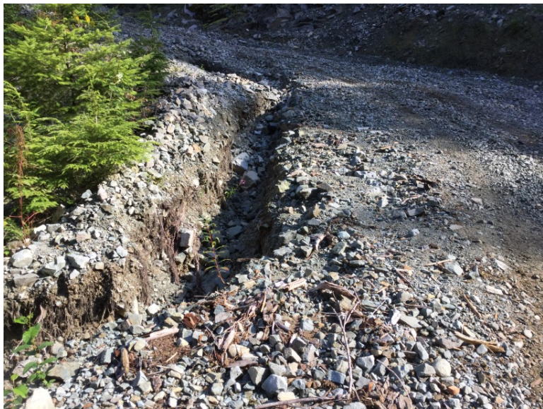
Running surface scour at right approach
