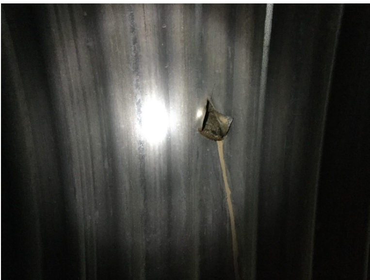
Culvert punctured from fill in 6 locations at left bank
